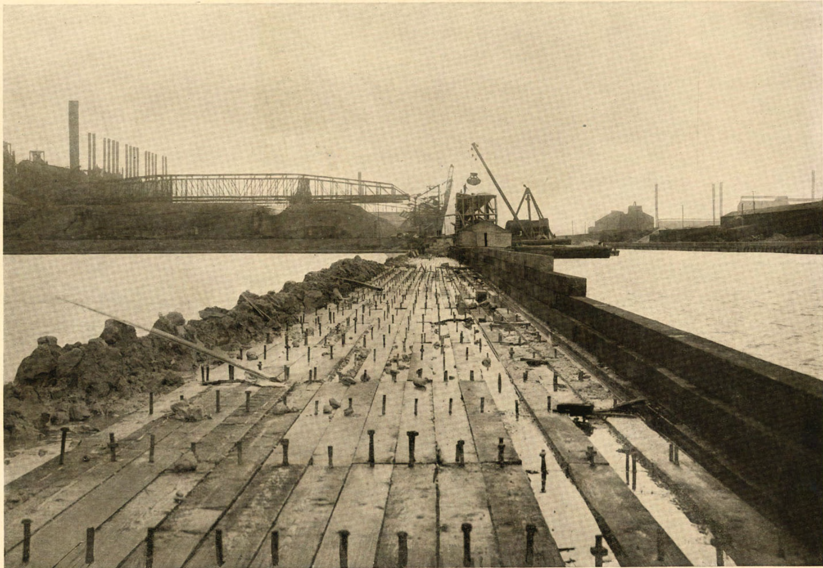
Mc SOUTH CHICAGO, ILLINOIS: Crib work ready for concrete superstructure, built for the Illinois Steel Company's plant on Calumet River.
